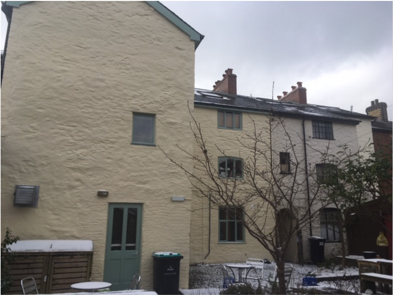
The rear of the building in winter 2020/21 following repair and renovation with the café still closed.
